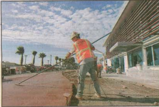
Concrete finisher Danny Stewart smoothed out fresh concrete in front of the new terminal at McClellan-Palomar Airport, which opens Nov. 17 as part of a $20 million renovation. Charlie Neuman / Union-Tribune
