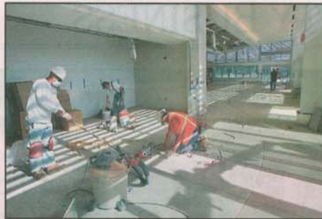
Workers finished the floors on the new $6.5 million terminal at McClellan-Palomar Airport recently.
